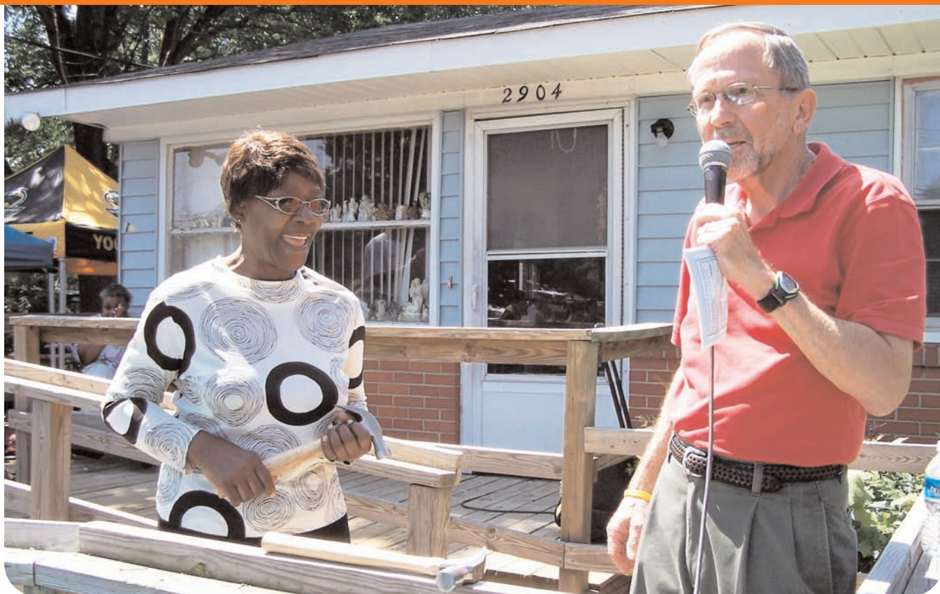
Bob Kelly of Housing Greensboro, right, kicks off repairs at the home on Phillips Avenue
